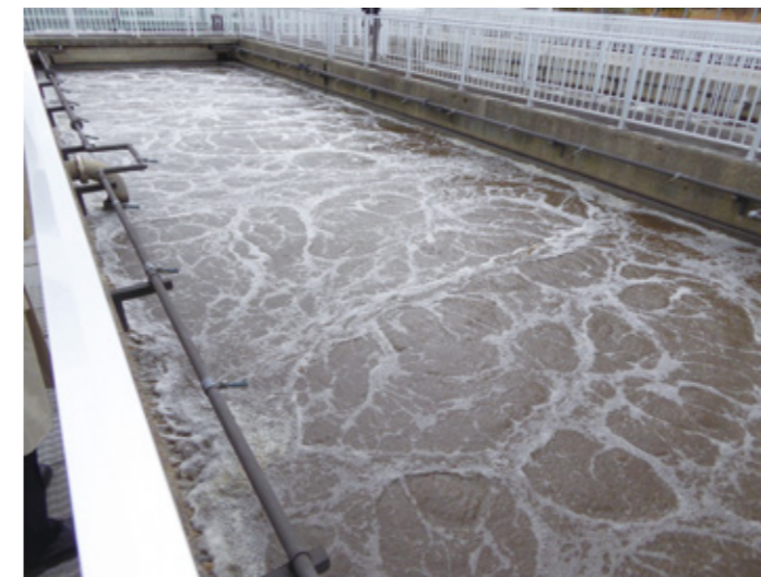
Fig.1 Activated sludge bioprocess in a sewage treatment plant.
