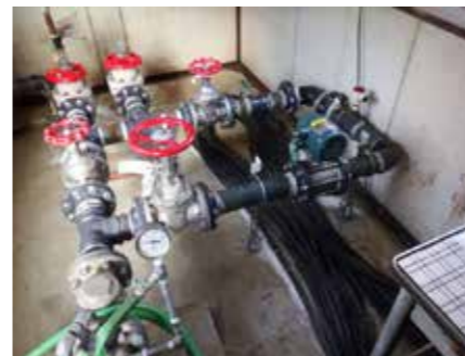
Fig.4 Monitoring system of hot springs for coexistence of geothermal power generation and hot springs
