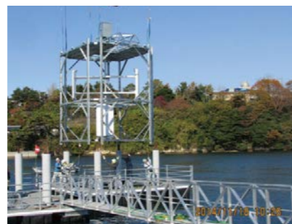
Fig.4 The tidal energy converter was installed by a crane ship (Sabusawa channel in Urato Archipelagos)
