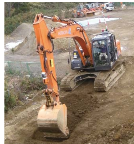
Fig.3 Soil excavation test by hydraulic power shovel with different soil strength characteristics.
