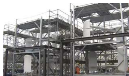
Fig.3 Assembly of the tidal energy converter (Local company in Shioyama :Tohoku Dock Tekko Corporation)
