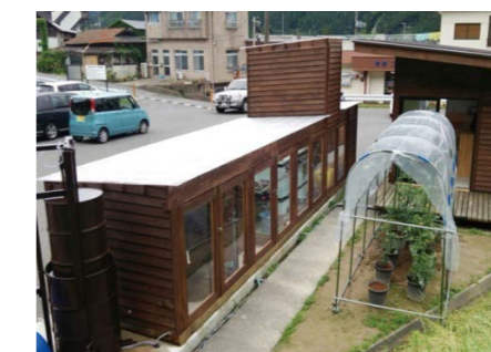
Fig.6 The compact & high efficiency methane fermentation system ( Yumeguri parking place in Naruko hot spring )
