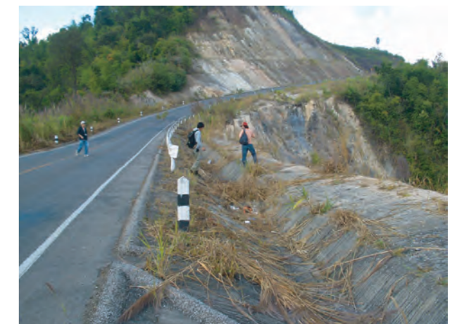
Survey of slope failure in the Northern Thailand caused by downpour
