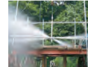
Multiple nozzle system for perforation at field.
