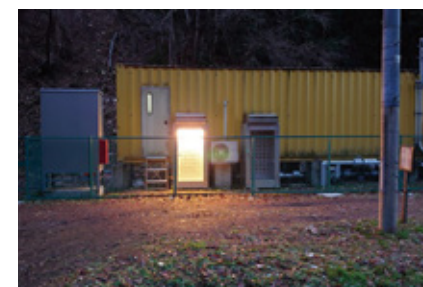
Fig.4 Field test of small-scale hot spring power generation system
