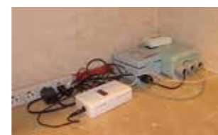
Development of H 2 S monitoring system
